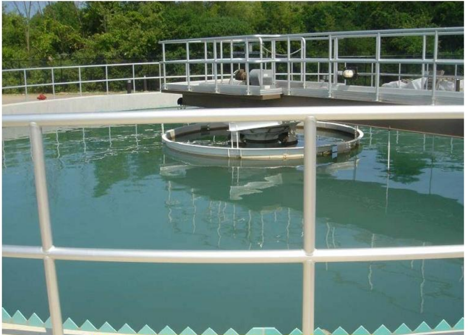
Figure 7 : Circular sedimentation Tank
